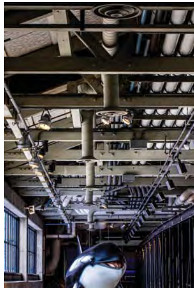
Mechanical Systems Monterey Bay Aquarium Chris Parsons
